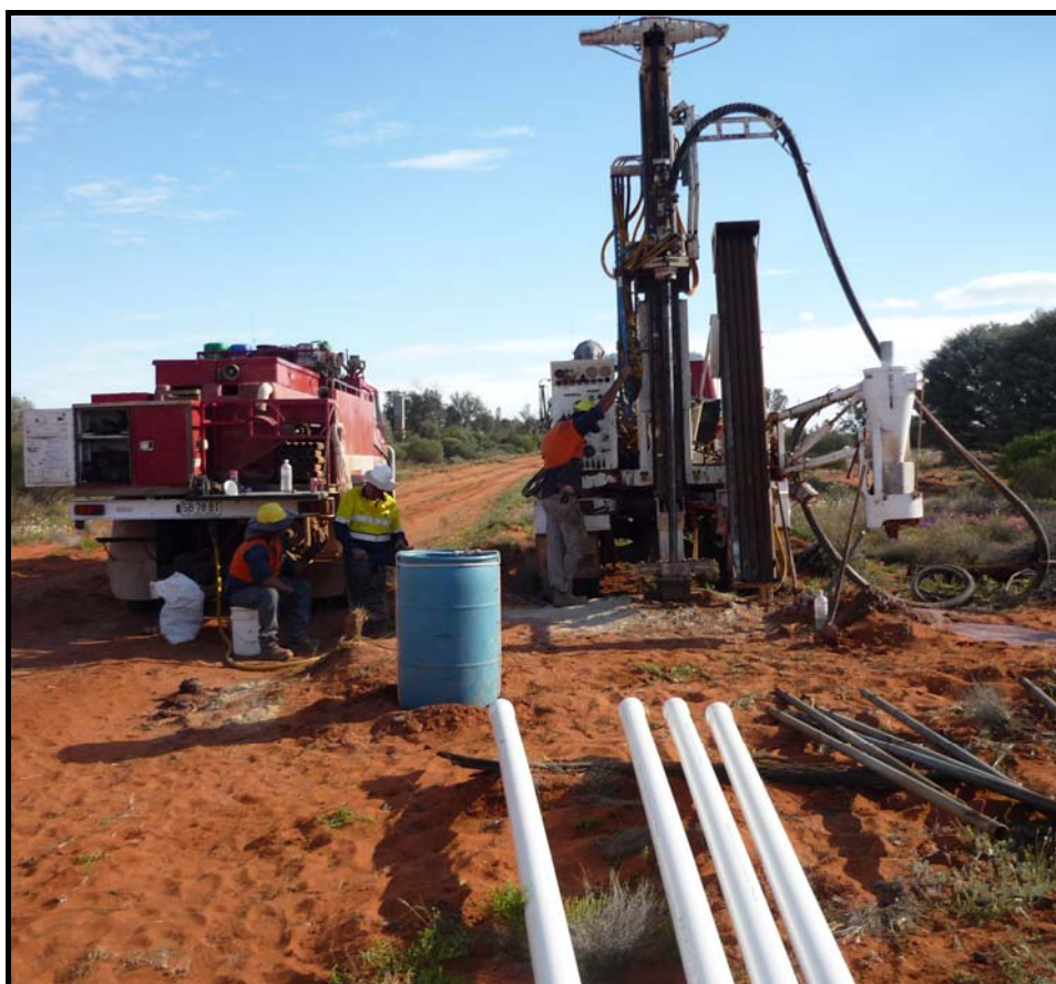
Shallow water bore drilling along access road to Cyclone using Diatreme's drill rig – September 2013
